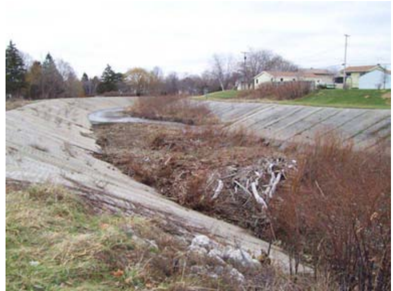
DEBRIS ACCUMULATION CONCRETE CHANNEL, 3000 LF
