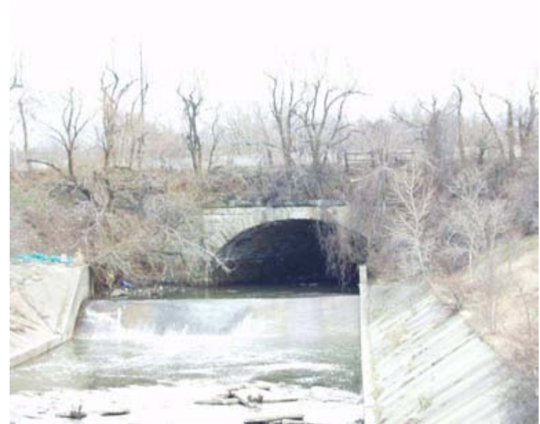
DAM IS BARRIER TO FISH MIGRATION AT RAILROAD
