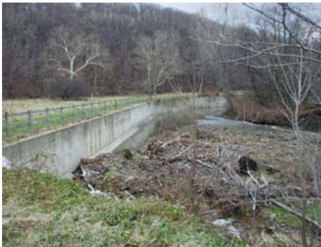
SEVERE BANK EROSION & CHANNELIZATION IN EUCLID CREEK RESERVATION
